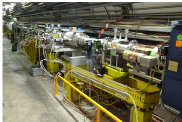
UA9 installation in the SPS
