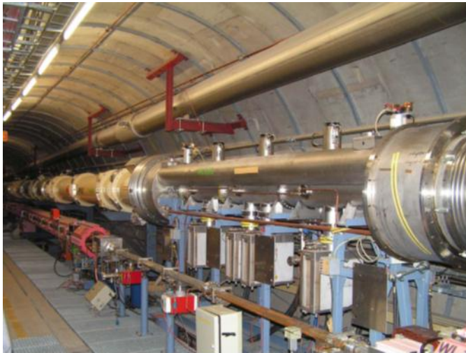
Kicker bypass line in HERA tunnel
