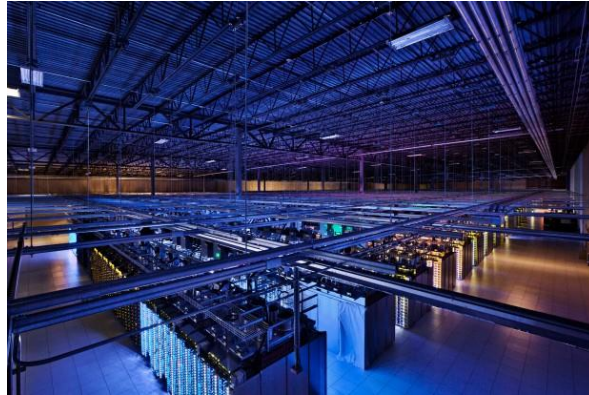
Google data center
