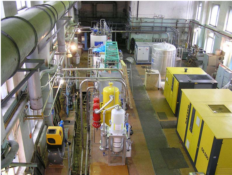
Hall of the cryogenic equipment
