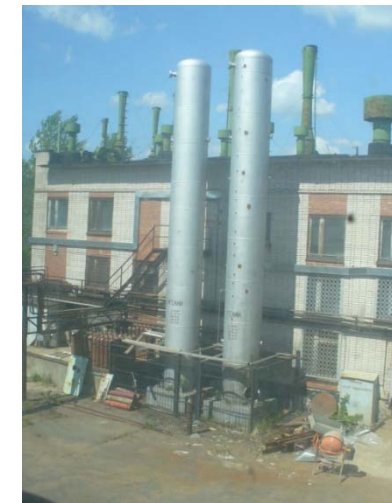
Receivers, cryogenic building
